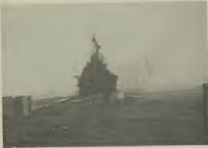
Fig.8.6 Effect of ground-shock from a buried bomb on a group of unreinforced brick surface shelters. The roof of the shelter on the left is seen separated from the walls while that next to it has its back broken by the movement. (Paragraph 8 & 31)
